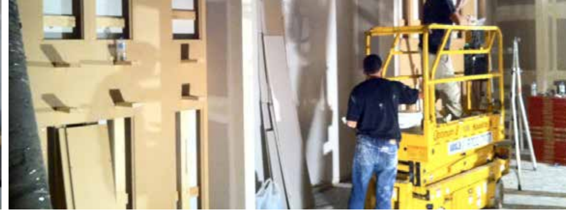
Biblos Highpoint Shopping Centre. Installation of a feature protruding puck wall system.
